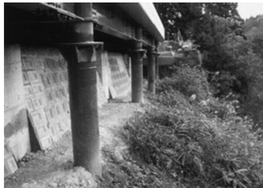
Photo 3 Sanada-Takashima Metal-Road after Niigata-Chuetsu Earthquake (View from slope side)
