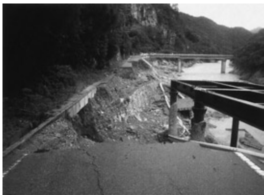
Photo 5 Metal-Road (under construction) after Typhoon 2004-21 at Mie Pref.
