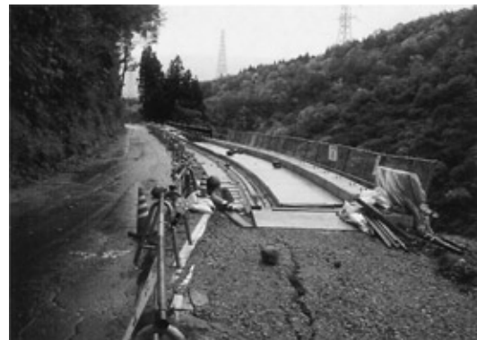
Photo 2 Sanada-Takashima Metal-Road after Niigata-Chuetsu Earthquake (View on road)
