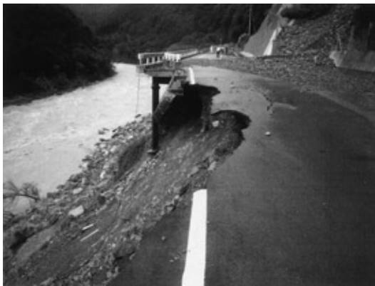
Photo 4 Metal-Road after Typhoon 2004-21 at Mie Pref.
