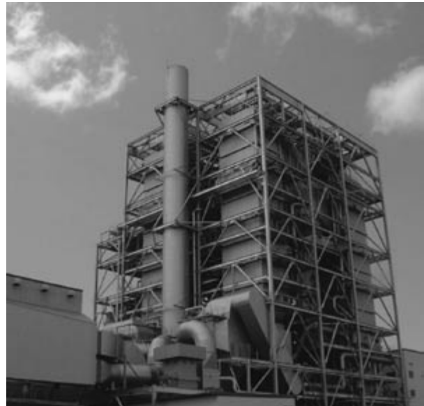
Photo 1 Appearance of boiler (rear view)
