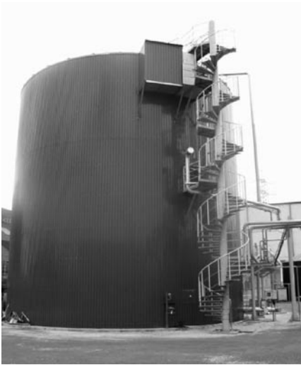
Photo 2 Digester at Chiba Biogas Center
