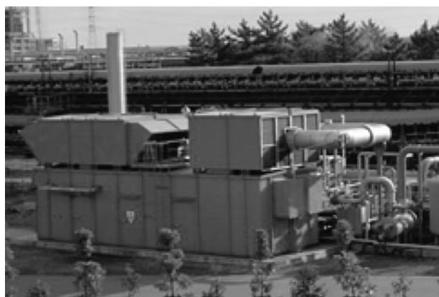
Photo 2 Gas motor generator
