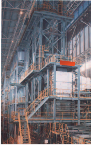
Photo 1 West Japan Works (Fukuyama) No. 3 Continuous Annealing Line (WQ-CAL)
