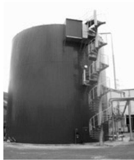
Photo 2 Digester at Chiba Biogas Center
