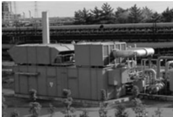
Photo 2 Gas motor generator
