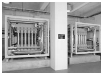
Photo 16 Tap water membrane filtration device
