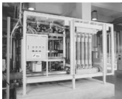
Photo5 Drinking water supply system using membrane treatment
