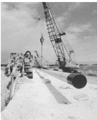
Photo 1 Natural gas pipeline
