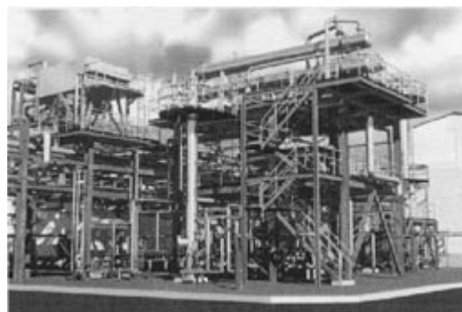
Photo3 Natural gas production and treatment facilities
