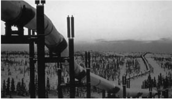
Photo 4 Scene of line pipe in operation
