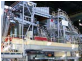
Ladle refining equipment
