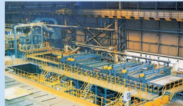
連続酸洗設備/Continuous pickling system
