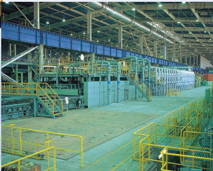
Heat treatment system
