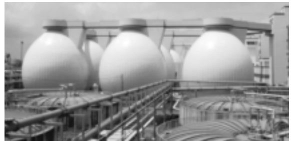
Photo 1 Egg-shaped sludge digestion tank in Yokohama Hokubu Sludge Treatment Center
