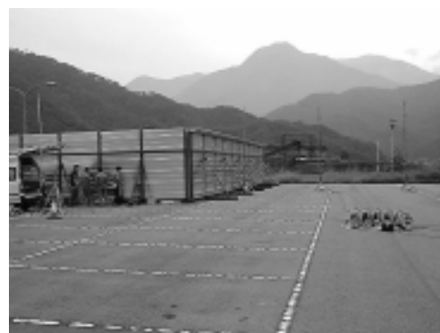
Photo 2 Whole of a noise barrier
