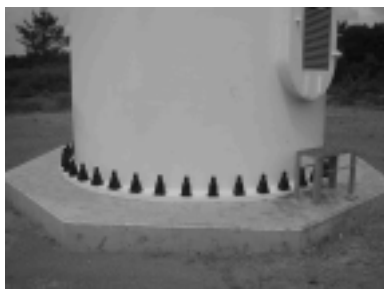
Photo 3 Protection caps for exposed PC anchor bolt's thread (Esashi)
