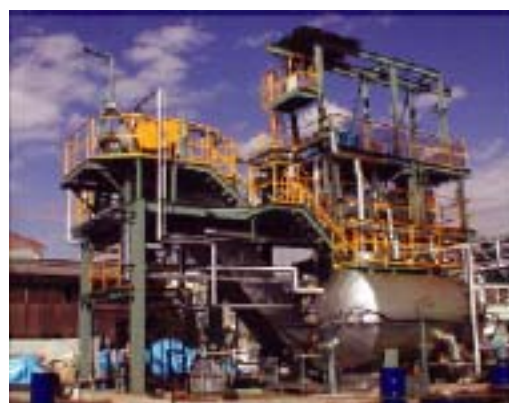
Photo 2 Outlook of pilot plant
