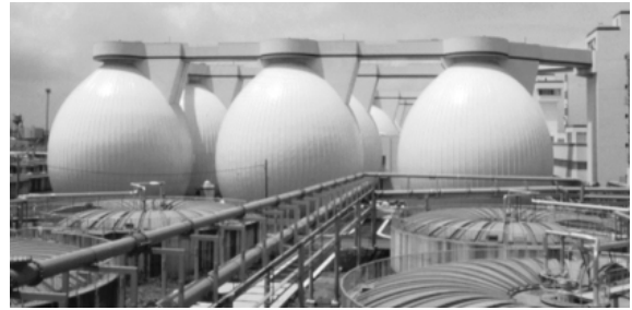
Photo 1 Egg-shaped sludge digestion tanks at North Yokohama Sludge Treatment Center
