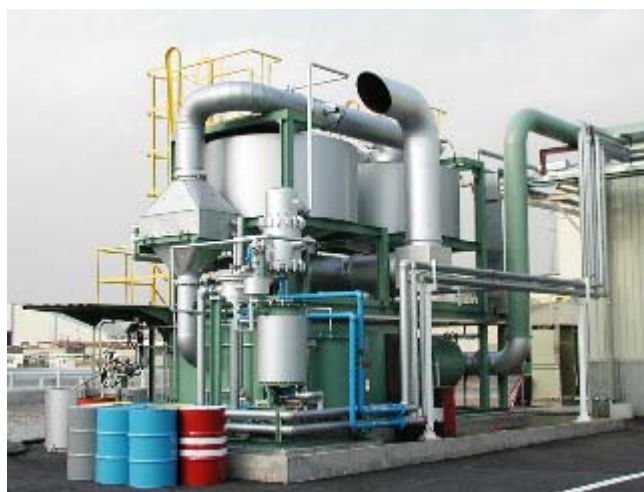
Photo 2 The facility for collecting chlorofluorocarbon from insulation material
