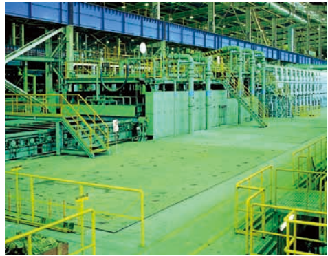
Heat treatment system
